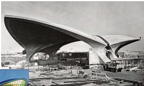
THE ROOF stands free of its complex scaffolding. A 1962 print ad, far left, shows the finished terminal in a dramatic light.
